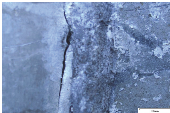
8: Failure of material next to the weld bead
